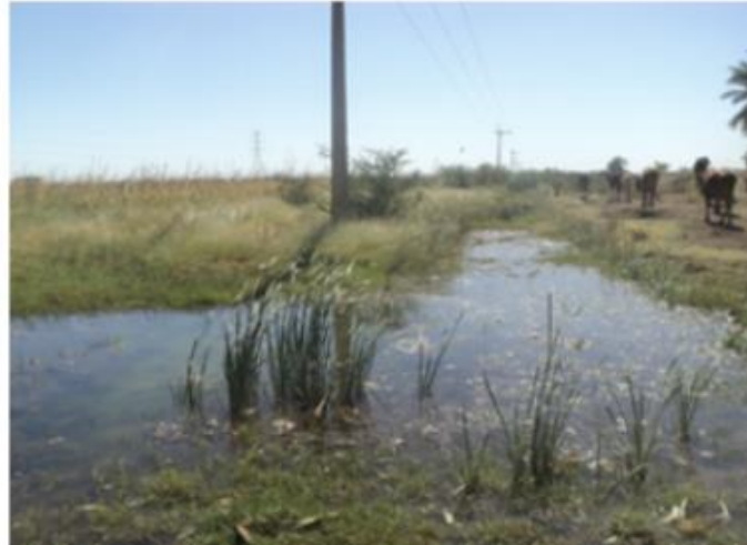
Fig. 2 Typical irrigation network infected by weeds and blocked by silts
