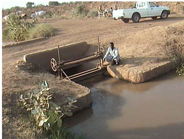
Fig. 6. Weeds and silts at movable weir opening (2.0 m)
