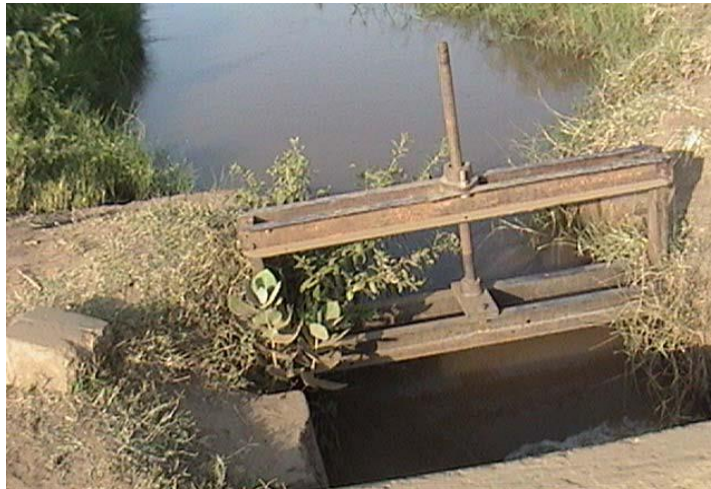
Fig. 5. Weeds and silts at movable weir opening (1.3m)
